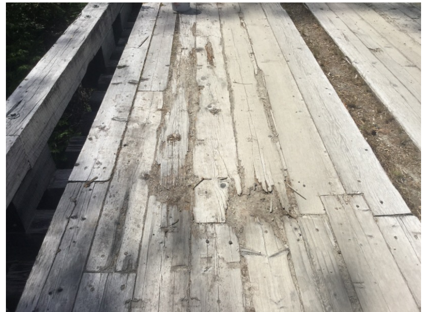
Pockets of Rot in Running Planks
