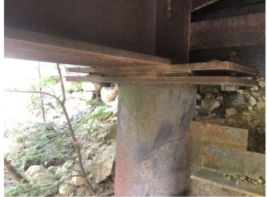
Right Abutment Downstream Bearing Bulging
