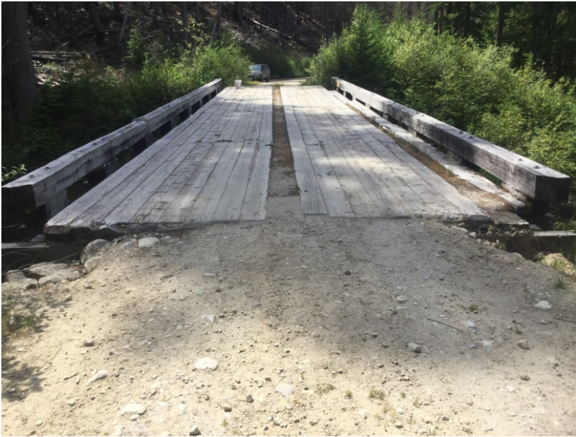
Poor Fill at Right Abutment
